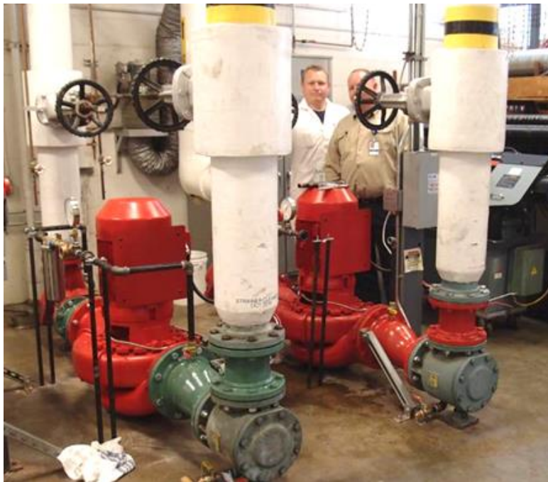
Figure 15 - Victoria General Hospital's new heating hot water pumps.
