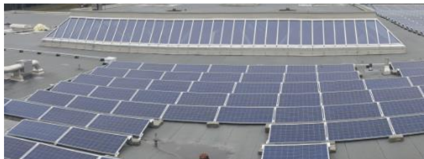
Figure 18 Solar Electric Panels at WCGH
